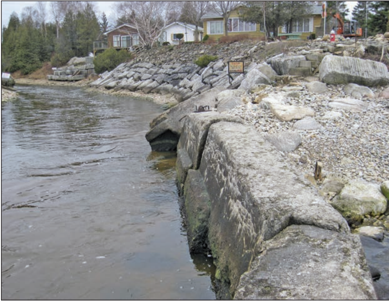
Photo: The bank of the channel at Barrow Bay leading from Georgian Bay to Little Lake. The channel has become shallow, narrow, and dangerous for boaters, requiring reconstruction of the break wall and channel dredging..
