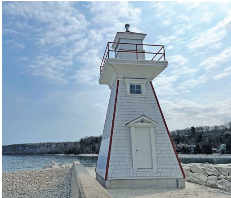
Photo: The newly built Lighthouse in Lion's Head. Proceeds from the fundraiser event on May 21st will help to further repair the most recent damage to the structure, shown on the bottom left of the lighthouse where a temporary patch has been placed.
