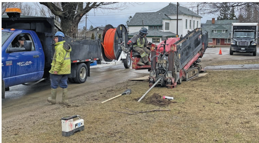
Photo: On 7 April 2022, a horizontal directional drill operated by Next Level Directional Drilling, laid fibre optic cable on John Street in Lion's Head.
