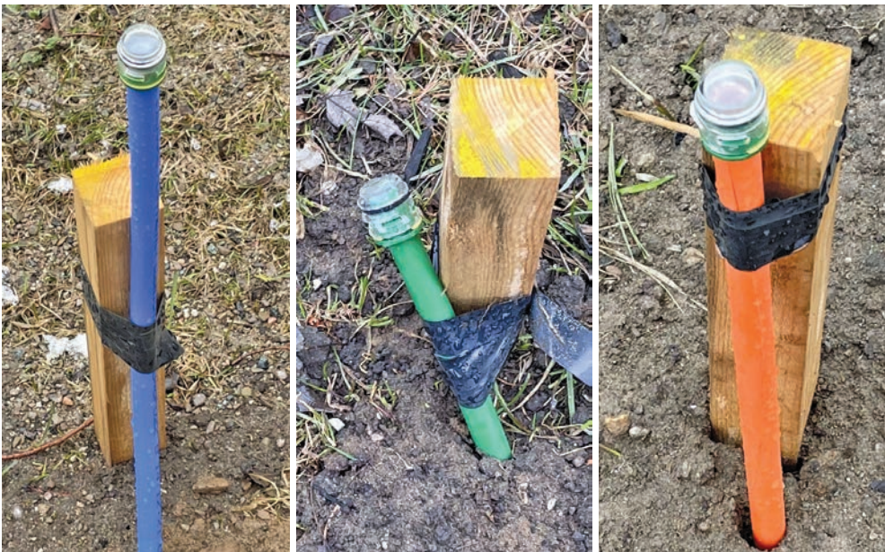
Photo: The different colours of conduit coming out of the ground are called '1 Way Microducts'. These are the 'drop' conduits that connect the main conduit line with each individual home/premise. These 'drop' conduits provide the pathway for the micro fiber optic cable to be installed between the nearest splice point and the premise. Once connected, these microducts will be buried and no longer visible in the boulevard.
