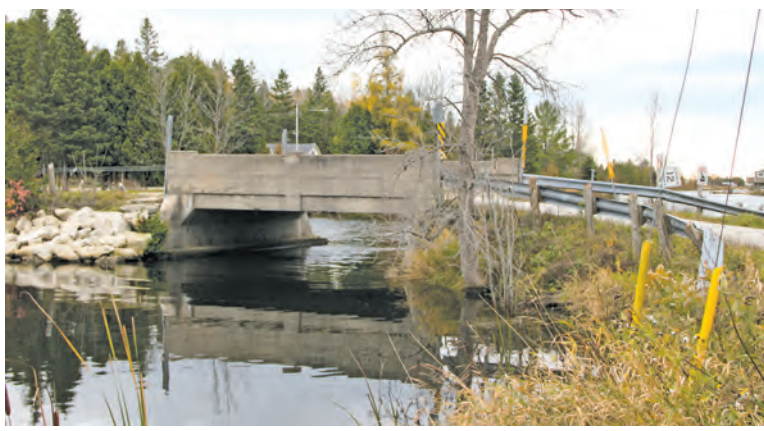
Photo: Heron Point Bridge looks fine above the water line, but its foundation has deteriorated beyond repair.
