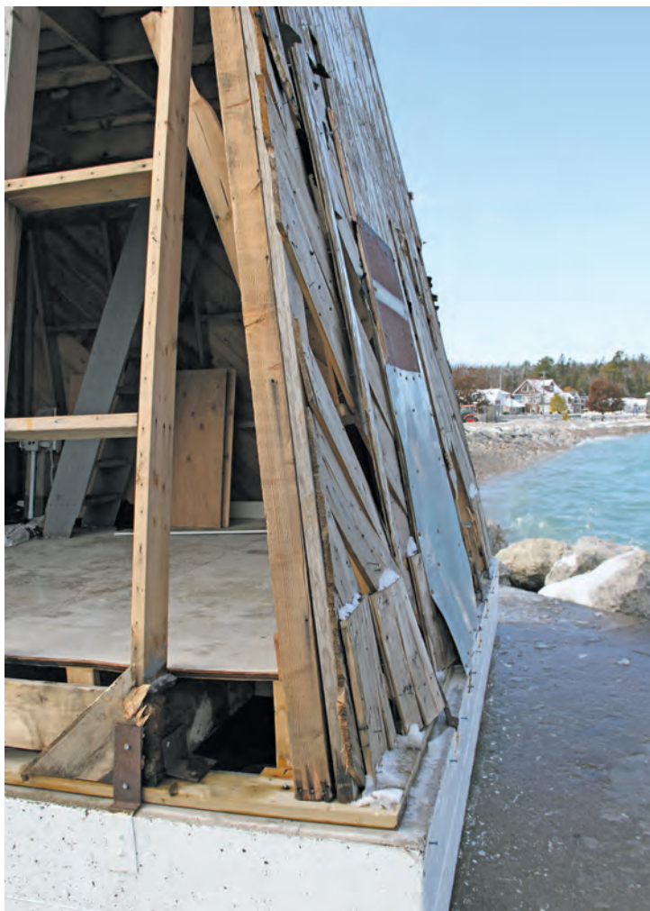
Photo: Close-up of the lighthouse shows the extent of the damage to the exterior.
