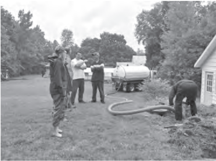
Photo: A.J. Arps from Bruce Peninsula Septic performs a demonstration at the previous Septic Workshop on July 17th.
